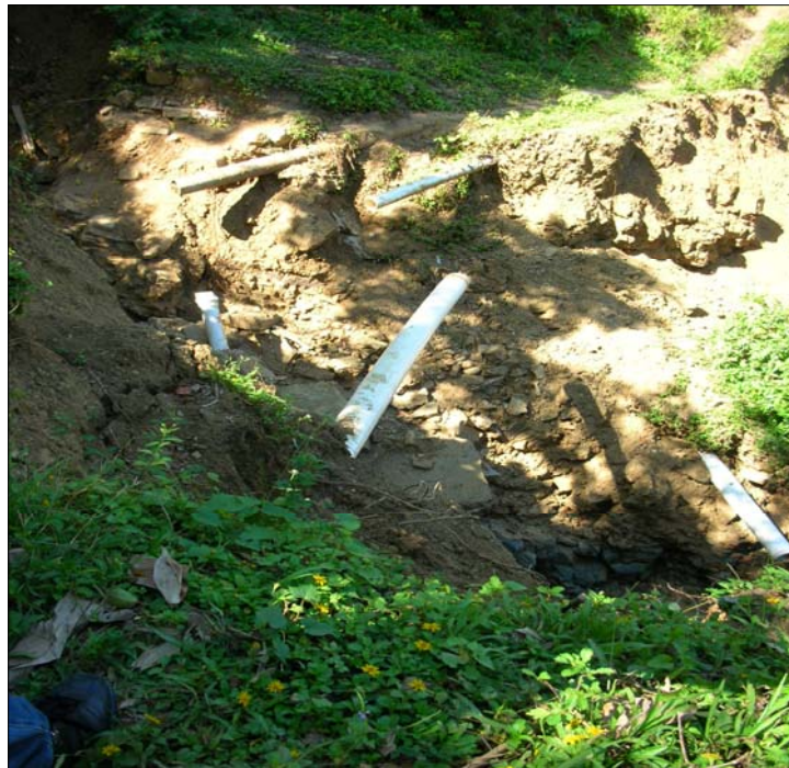
FIGURE 1. A break in one of the pipelines leading to Port-de-Paix.
