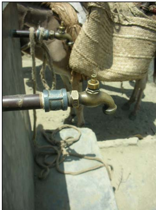
FIGURE 2. A non-functioning public fountain in Port-de-Paix being used as a tethering stand for donkeys.
